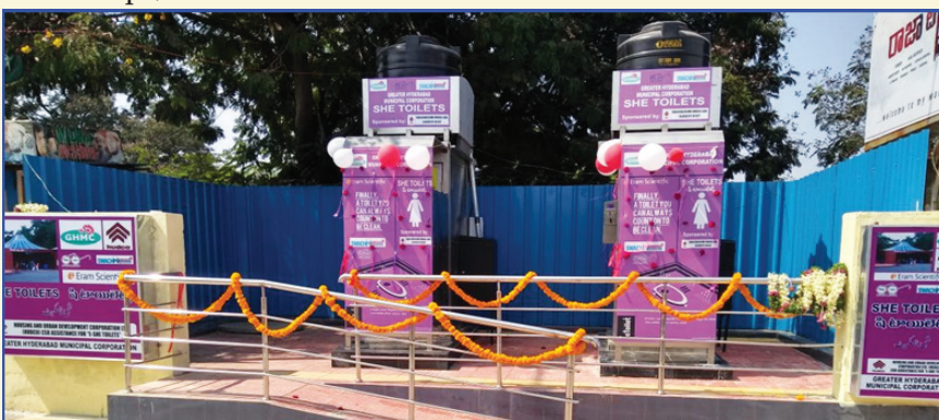
Installation of E toilets with SHE accessories in 15 locations in Greater Hyderabad Municipal Corporation (GHMC) limits, Hyderabad, Telangana State
