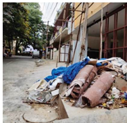
Figure 4: Construction debris on the public sidewalk alongside the construction site, Vijayanagar
