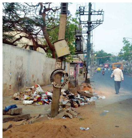
Figure 2: Garbage dump alongside a high boundary wall of a government institution, Magadi Road, Bangalore
